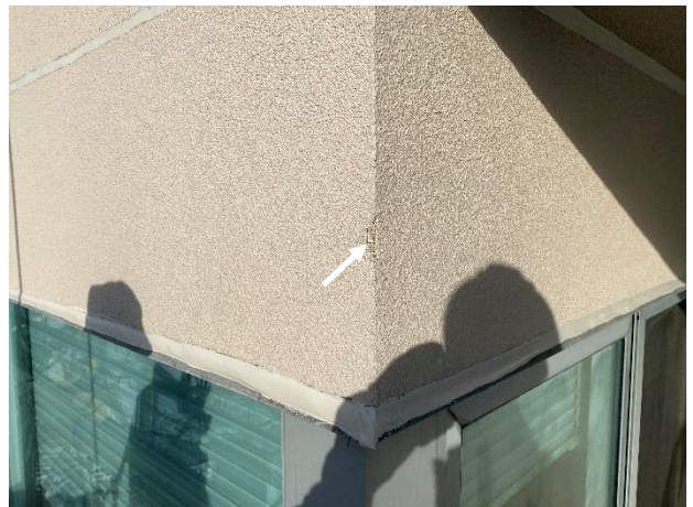
Damaged stucco finish at Suite 1203.
