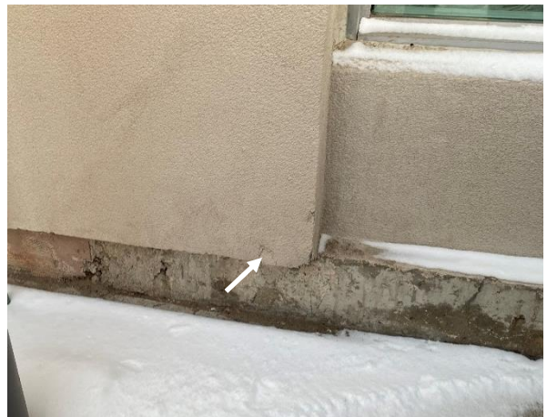
Example of outstanding patch repair.
