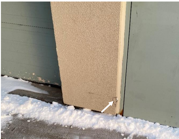
Example of outstanding patch repair.
