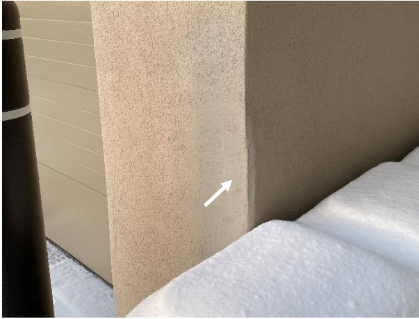
Example of inconsistent stucco finish.
