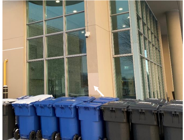
Area of incomplete coating work.
