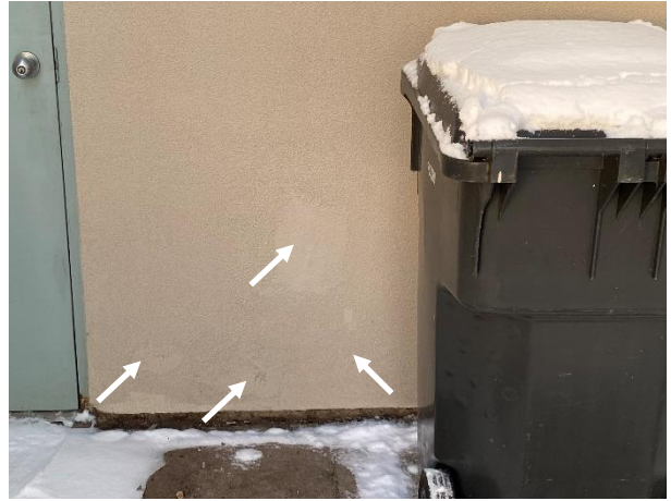
Example of inconsistent stucco finish.
