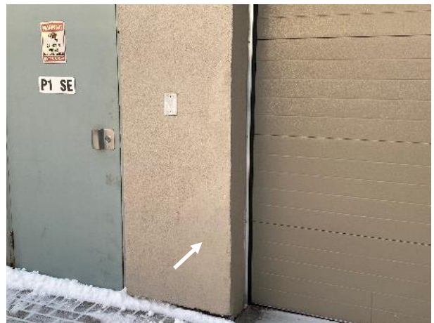
Example of inconsistent stucco finish.
